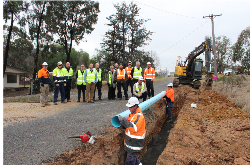
The first pipes being installed for the Scone to Murrurundi pipeline, 12 August 2019
